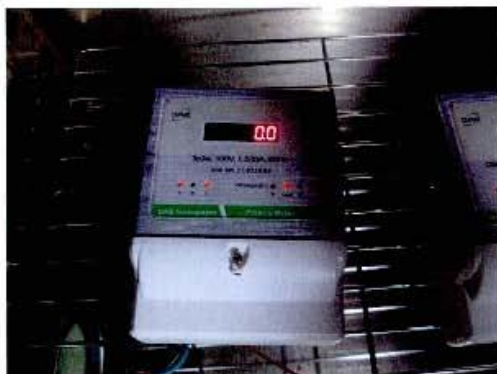
Figure 6 : 3p3W, 100, 1.5(6)A, 50Hz (Final condition)
