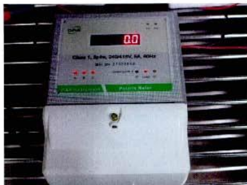
Figure 8 : 3p4W, 240/416V, 5A, 60Hz (Final condition)
